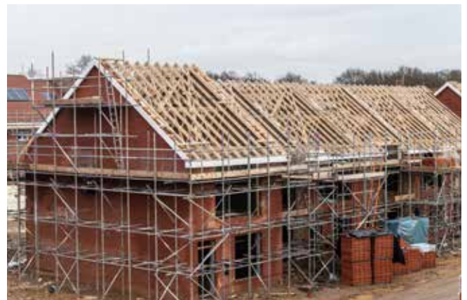
Figure 1: Sound insulation must be considered throughout the building process for new homes
