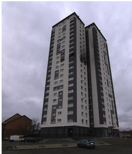
Figure 3 – Block of flats showing limited damage to the non-combustible cladding system after a fire
