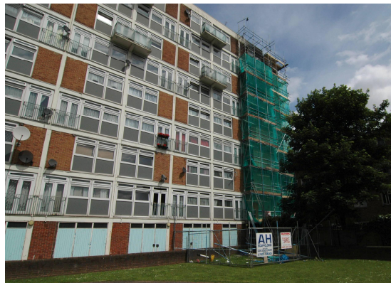
Figure 1 – Block of flats showing undamaged window sets; the fire damage is behind the scaffolding
