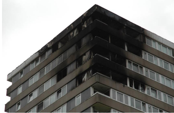
Figure 2 – Block of flats showing extent of fire damage caused by holes in compartmentation on balconies
