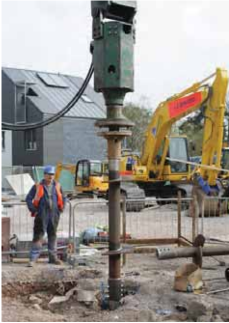
Figure 2: Helical steel (screw) piles being installed on the BRE Innovation Park, Watford
