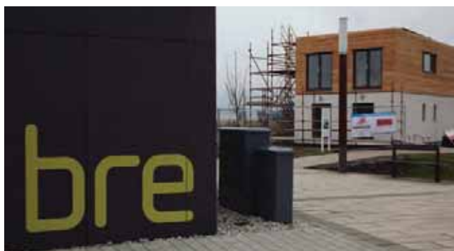
Figure 2: A low-energy demonstration home under construction at the BRE Innovation Park, Ravenscraig
