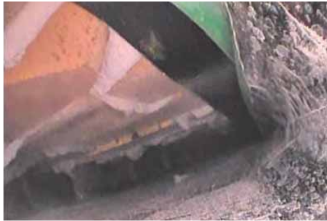
Figure 3: Videoscope view of the cavity behind the external façade. The fire stopping (green plastic membrane) is visible at the top of the photo
