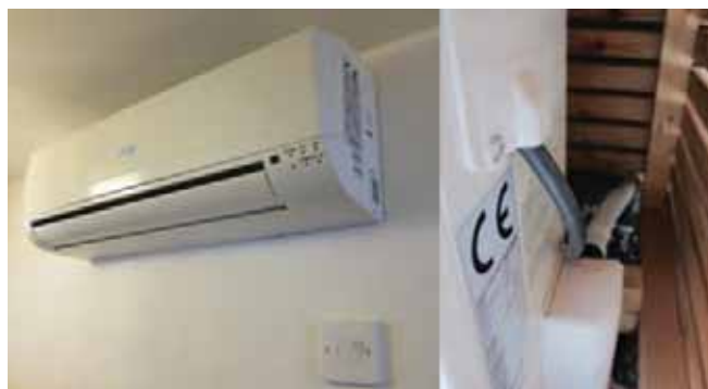
Figure 5: Air source heat pump located in dwelling built to PassivHaus standards. IDEAS tool could be used to highlight where novel control strategies could improve the performance of this heating system © www.flickr.com/murphygb
