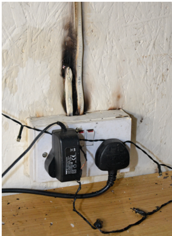
Figure 4: Example of a fire due to an electrical cause (photo courtesy of SFRS)
