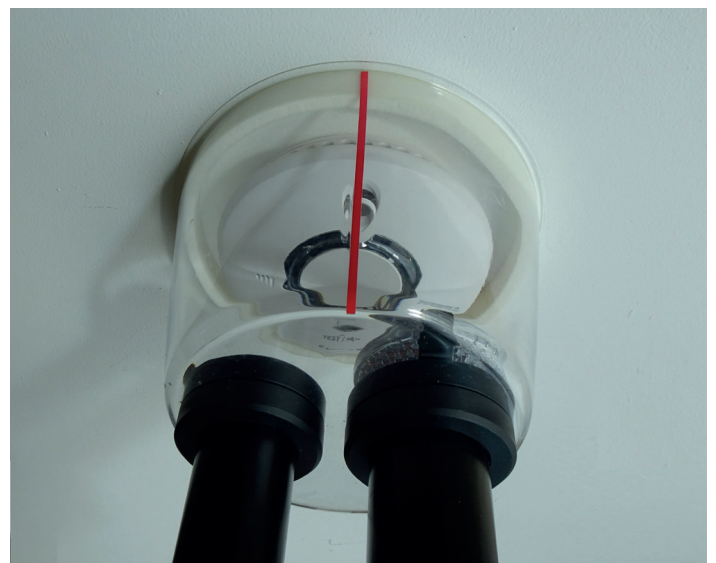
Figure 12: Trutest being used to test a domestic smoke alarm
