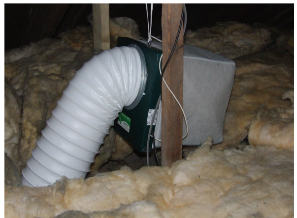
Figure 1: Roof-located positive ventilation system
