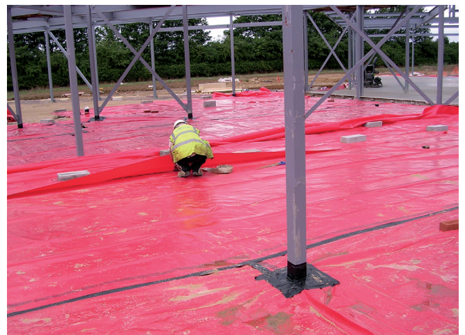
Figure 1: General view of a radon barrier laid over fill and sealed to columns
