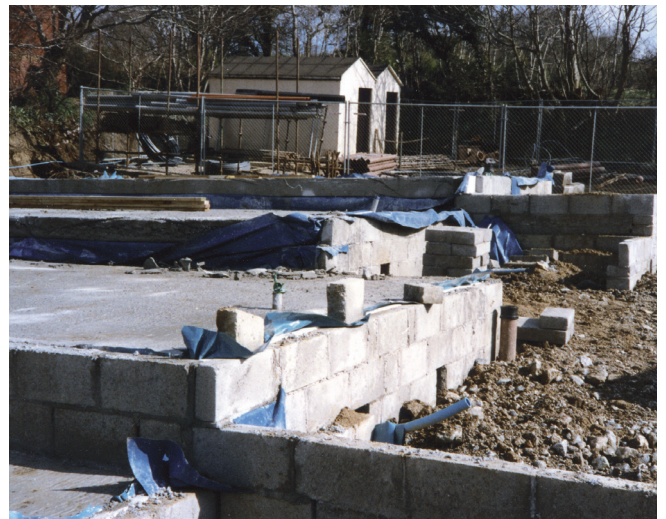
Figure 1: Steps and staggers in construction make it difficult to provide a continuous radon barrier
