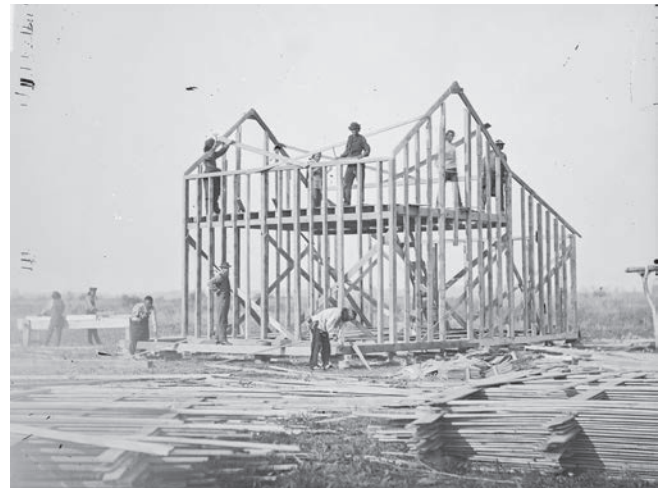
Figure 1: Construction of a balloon frame house in the United States in 1877 (photograph by William Henry Jackson; ©The National Anthropological Archives, Smithsonian Institution)
