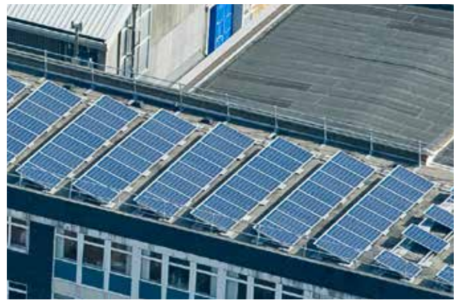
Solar PV installation at the BRE Group site at Garston
