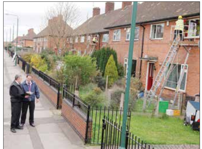
Figure 1: Decent Homes work in progress: installation of double-glazed windows. Photo courtesy of Nottingham City Homes
