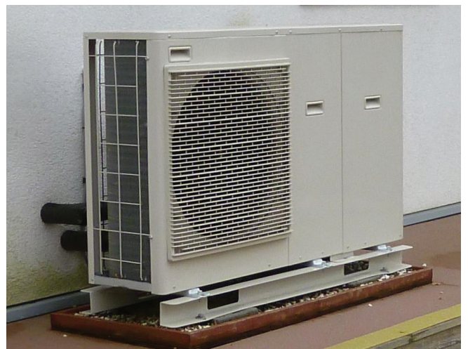
Figure 1: Air source heat pump installation on the BRE Innovation Park
